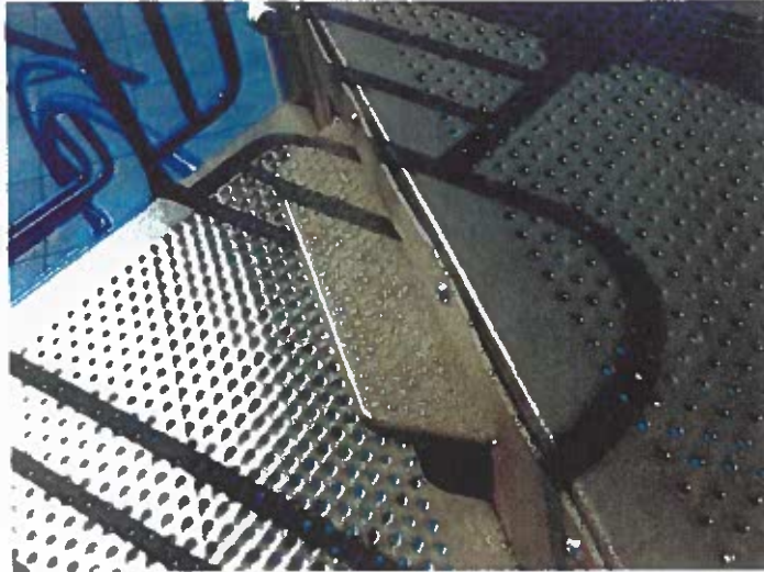
Intermediate Panel Pinch Hazard
