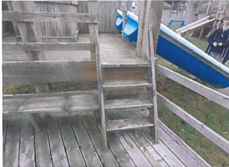
No Handrail on the Set of Stairs
