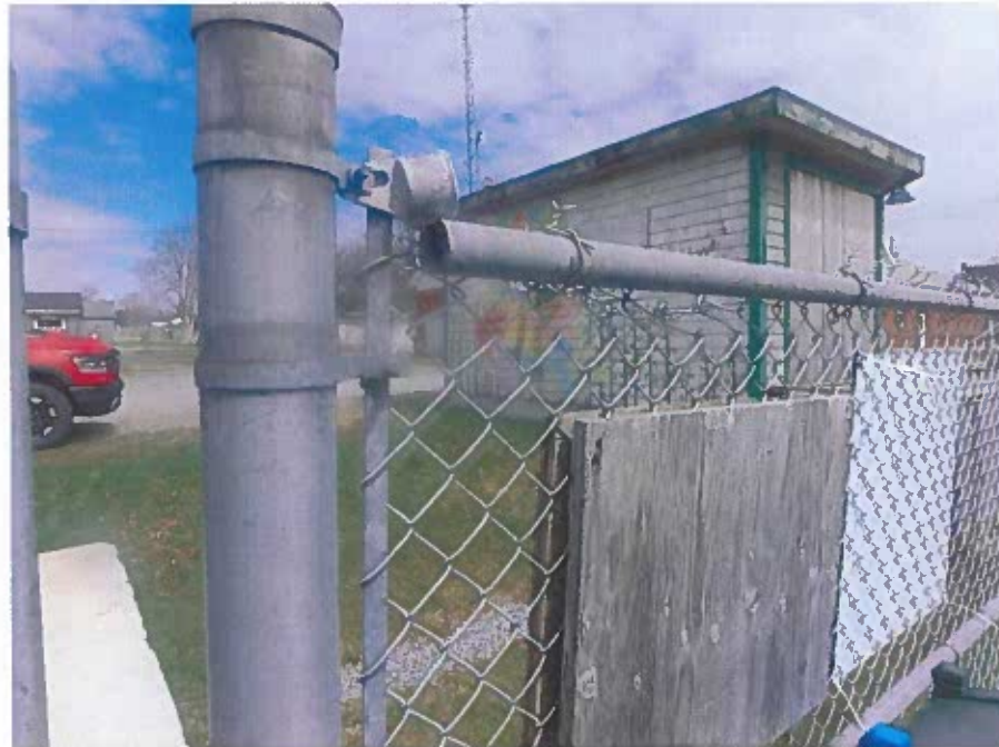
Disconnected Frame Pieces
