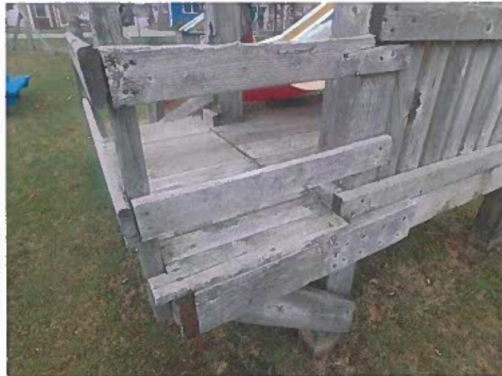
Torso Entrapment Hazard
