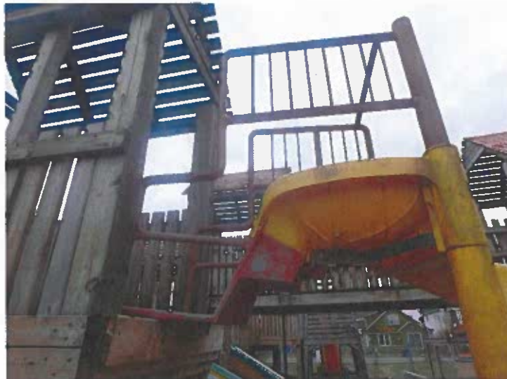
Non-Standard Openings on Guardrails at Top of Spiral Slide
