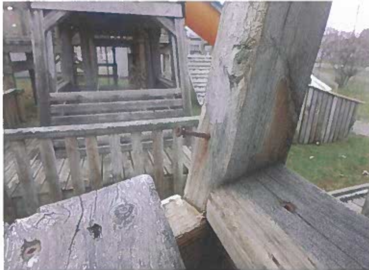
Protruding Screw on Structure
