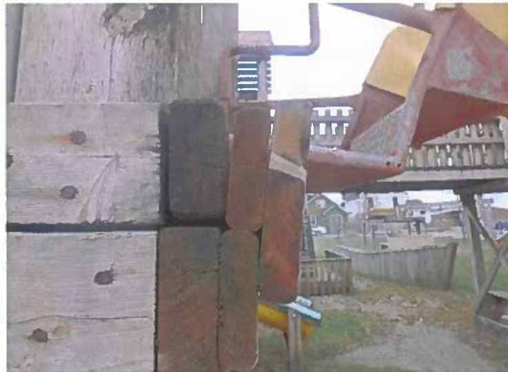
Wood Member Beginning to Detach at Spiral Slide Area
