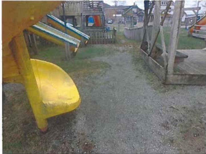
Non-Standard Clearance to Structure at Front of the Spiral Slide
