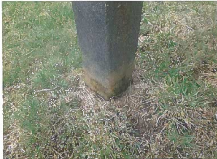
Rotted Wood Columns
