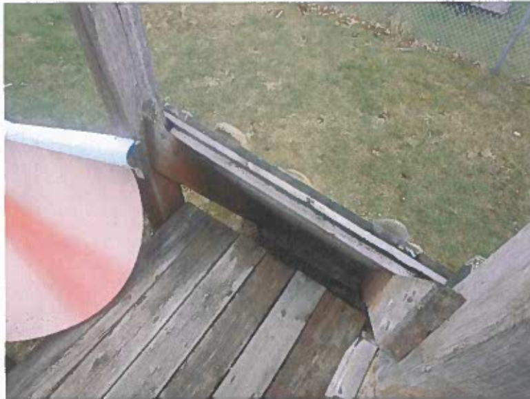
Rock Climbing Ramp Not Flush with Platform Surface
