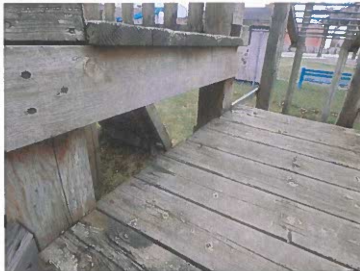
Torso Entrapment Between Platforms
