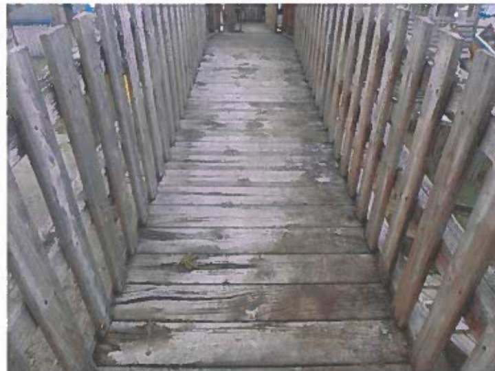
Some Rotted Deck Boards on Structure
