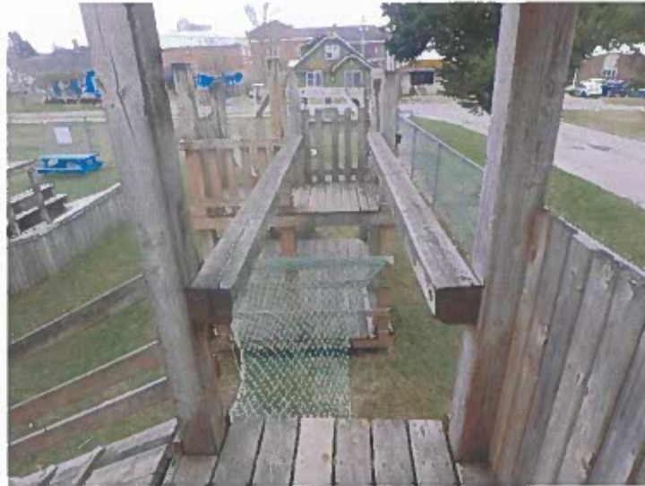
Open Guardrail Above Hammock Netting
