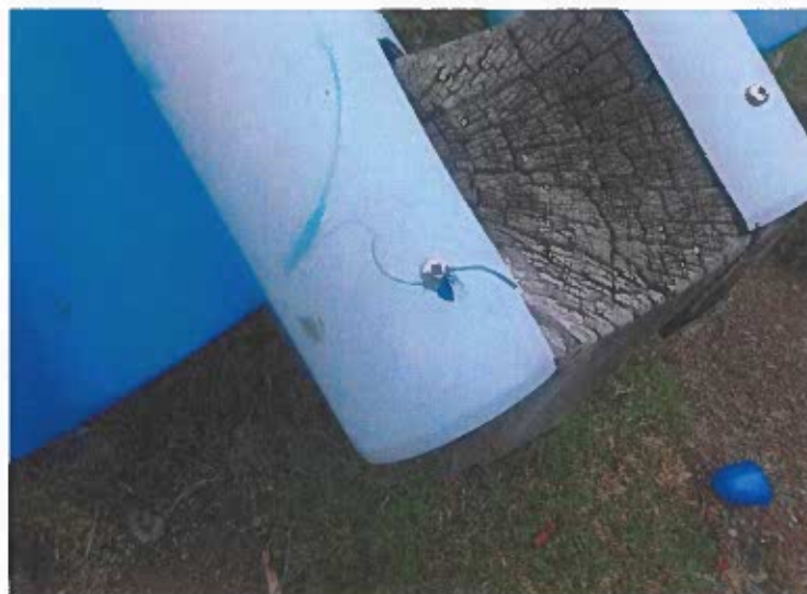
Cracked Slide Bed at Bottom Frame Connection
