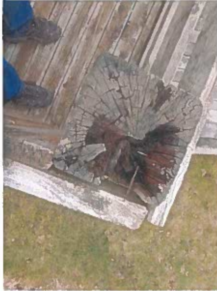
Rotted Wood Columns on Structure
